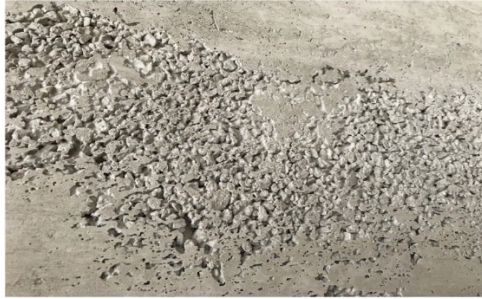
Figure 1: unacceptable substrate honeycombing
