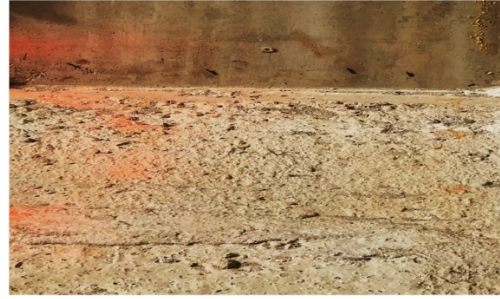
Figure 2: unacceptable substrate concrete protrusions
